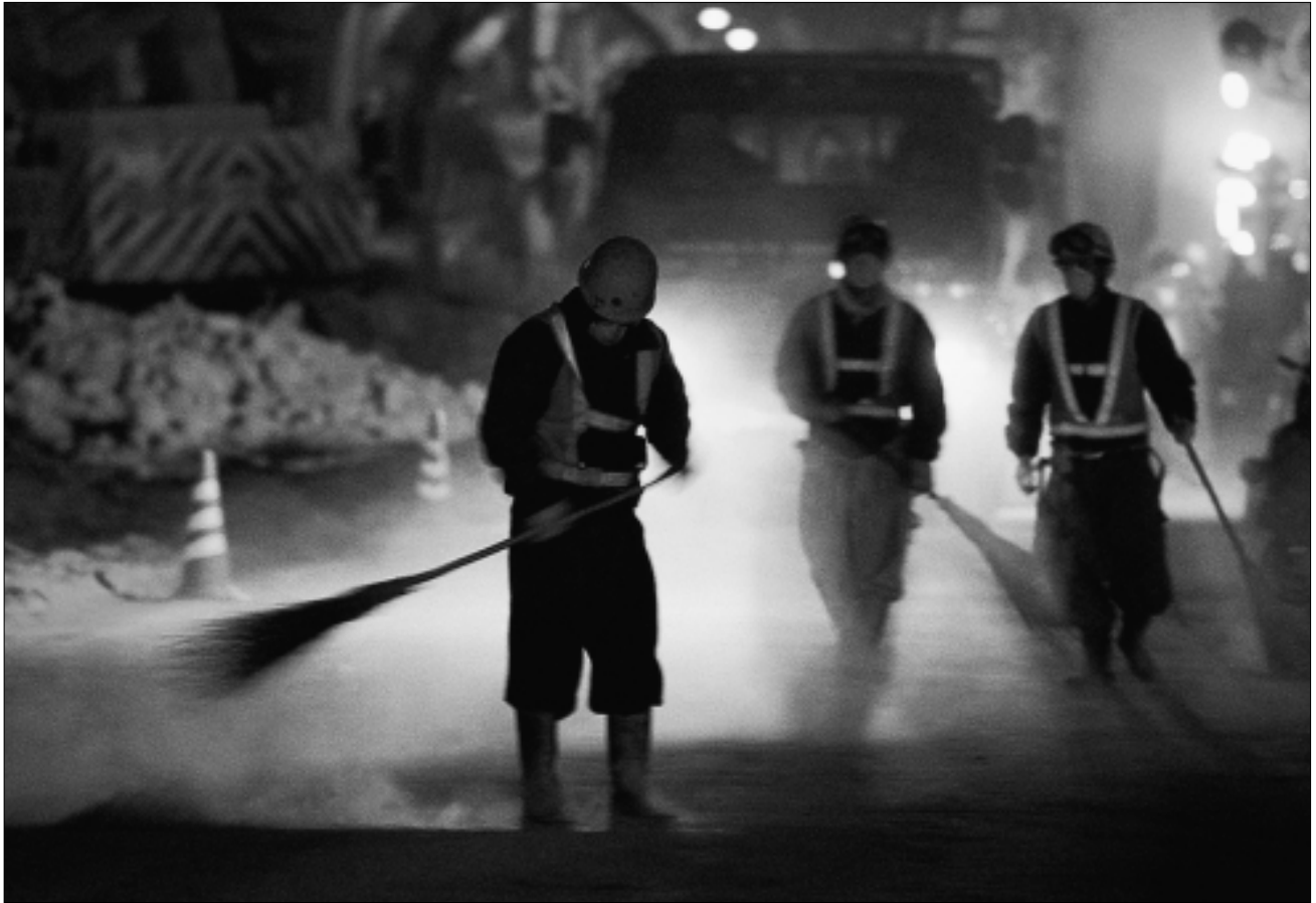
1:00 a.m.: Sweeping up after the Kobe earthquake, Japan.
