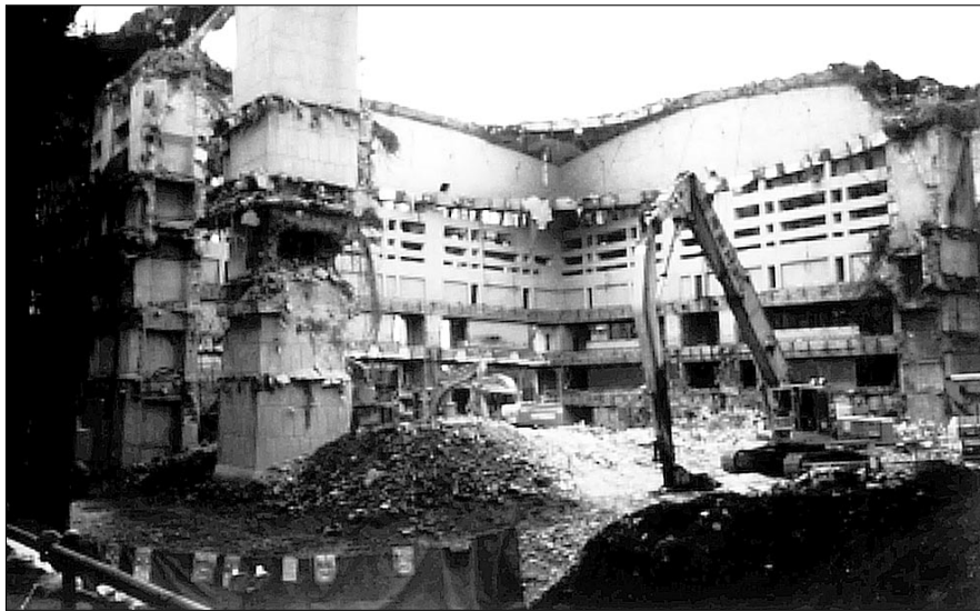
Nikken's reasoning that 'refuting slander' is why he's tearing down the Grand Main Temple calls into question his real reason for cutting down Gakkai-donated cherry trees and demolishing the Grand Reception Hall.
