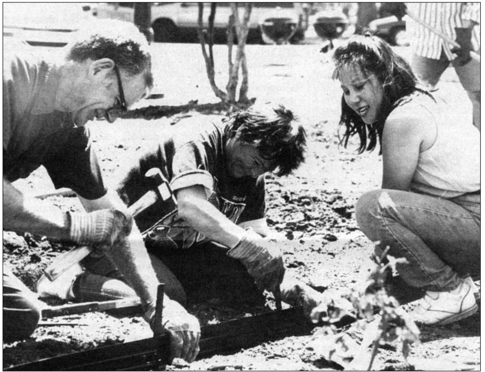
Volunteers install aluminum edging for the new pathways, during stage two of the project.
