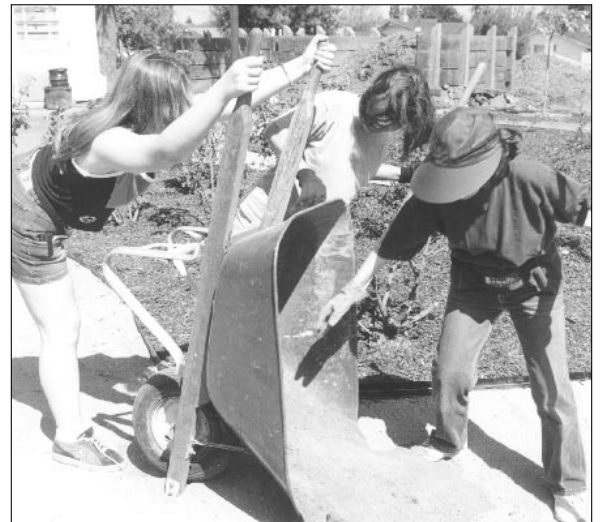
Laying sand and gravel on the new pathways. The weekend project involved removing four inches of soil for the new paths as well as old rose bushes and trees. An irrigation system was also installed.
